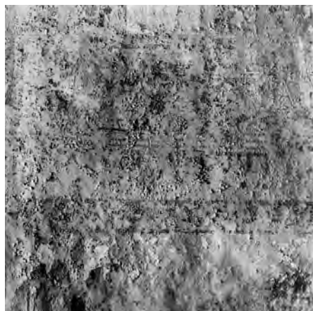
FIGURE 4 Flaking on the east wall of cave 85 (1973).
